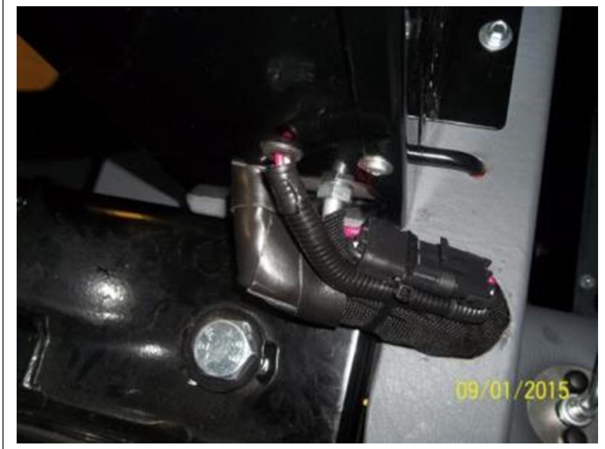
Hoses and wiring neatly wrapped.
