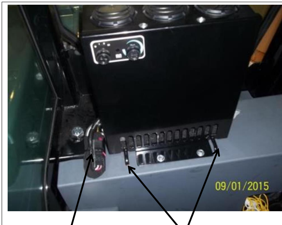
Hoses and electrical down here and into engine compartment.
